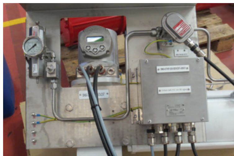
Figure1: Control Panel Low Pressure
