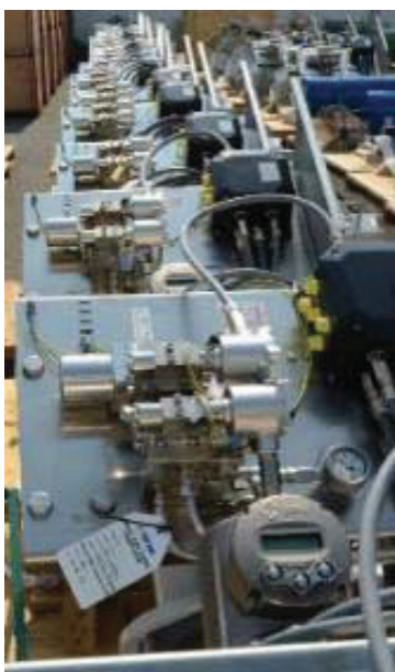
Figure7: Hydraulic High Pressure Control Panel
