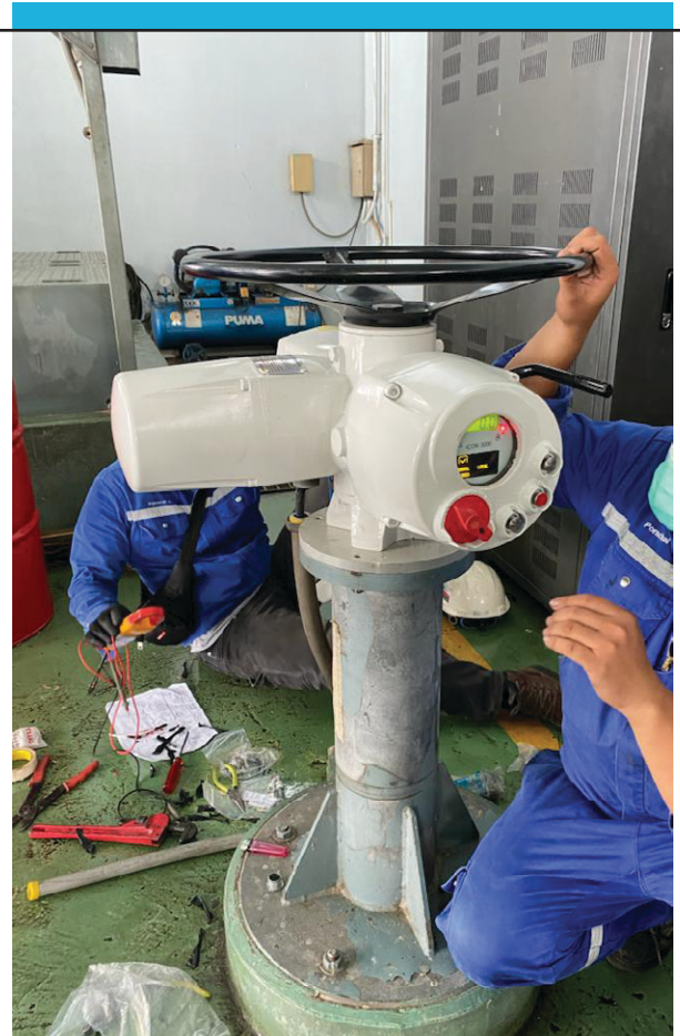
Biffi ICON3000 installed at a water supply transmission site
