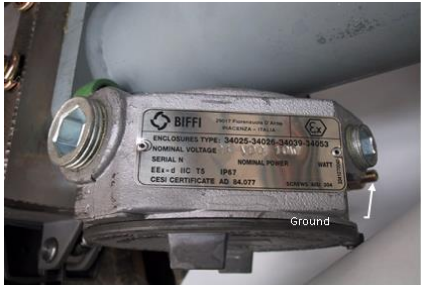
Picture 2 – Junction box on Control group
