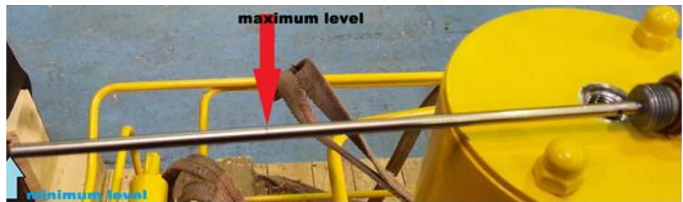
Picture 13 – Level measuring stick
