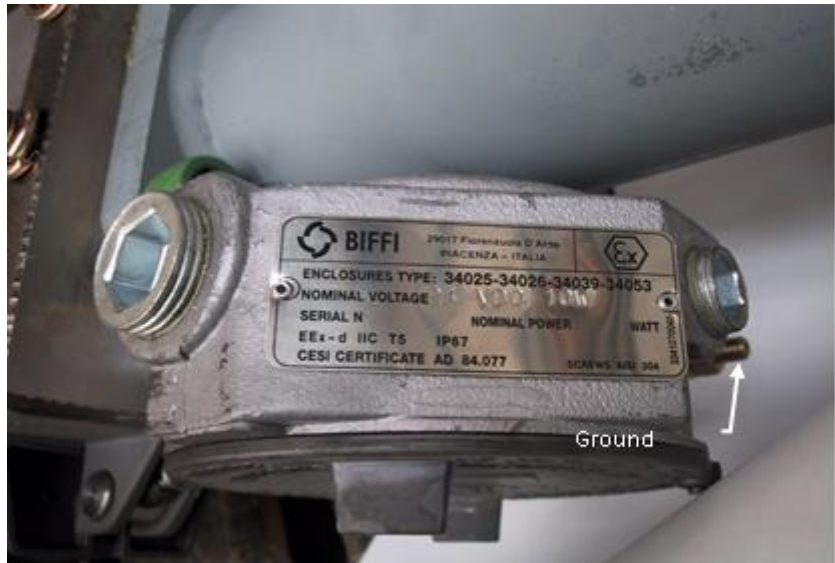
Picture 2 – Junction box on Control group
